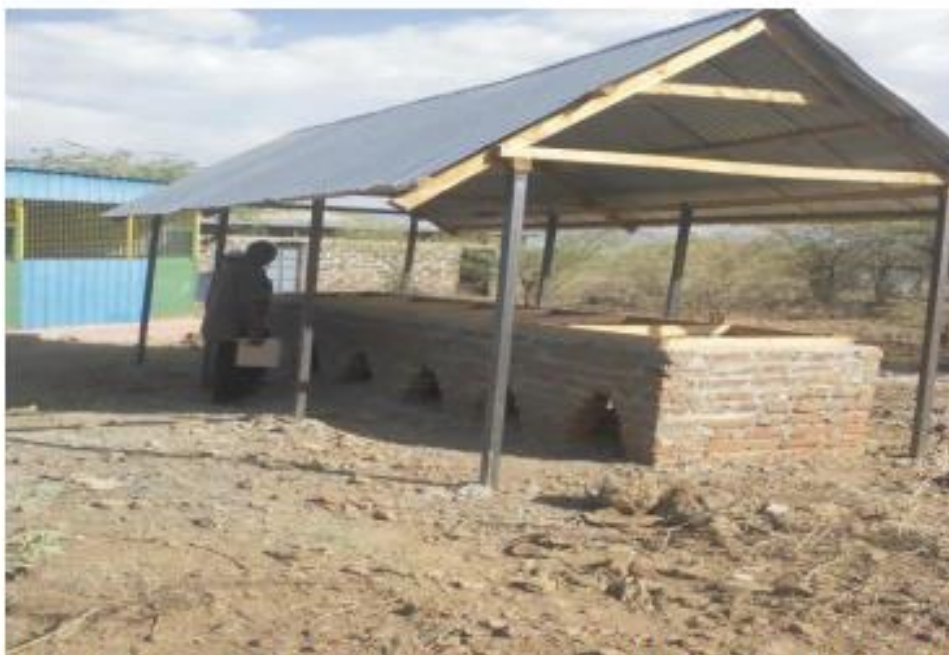
Plate 2. A five door Chorkor Oven smoking kilns installed by KMFRI at Kampi ya Samaki along Lake Baringo
