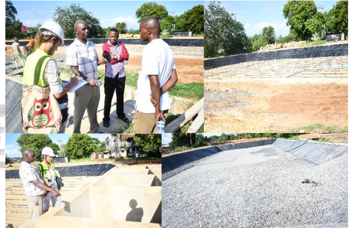
KMFRI senior research scientists Mr. Steve Mwangi and Dr. Joseph Kamau with the project consultant Ms. Sarah and site managers during a site tour of the wastewater treatment system in Shimo La Tewa Prison. The plant will facilitate the recycling of wastewater from prison and neighbouring social joints, houses, and private villas, whose sewage is discharged to Mtwapa creek every day, posing a health hazard to people and sea creatures. The recycled wastewater will, among other uses, be used for farming |Photos by Jane Kigita
