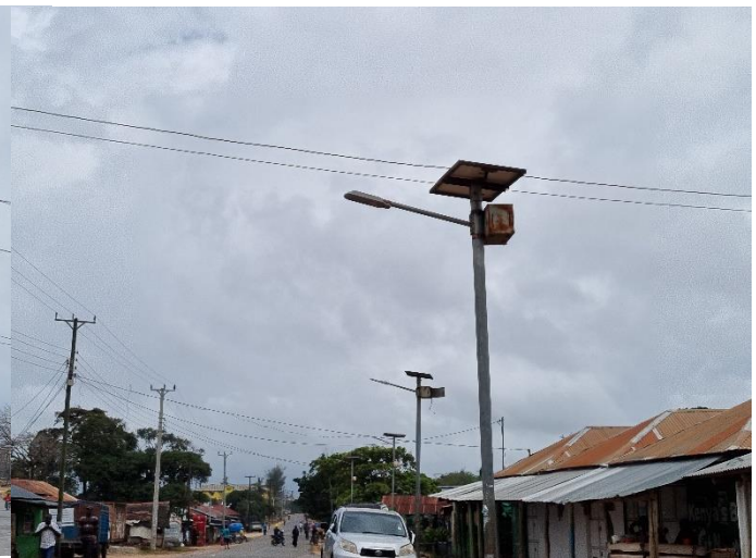
Plate 4-17: The market Centre is lit by Solar street lights
