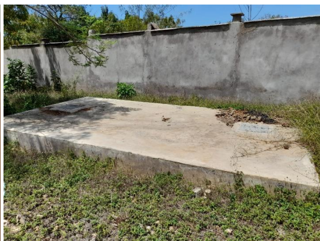
Plate 4-15: The septic Tank Serving the Administration block at KMFRl Shimoni NAMARET site
