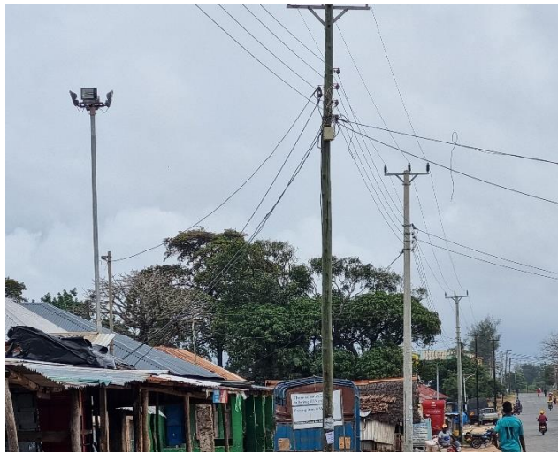
Plate 4-16: Shimoni Market connected to National Power Grid
